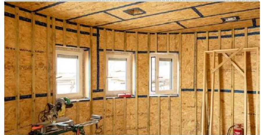
A good airtightness strategy forms the basis of an airtight building. This is an excellent example of taped OSB, with a dedicated service cavity on internal walls. The service cavity means most wires and pipes will not breach the airtight OSB layer.
